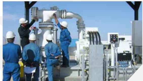
Training and Maintenance On-site Cost-effective and immediate
